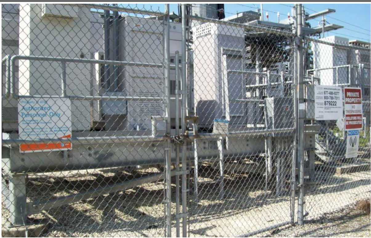
Site 36: Cell Tower with Diesel Powered Emergency Generator B
