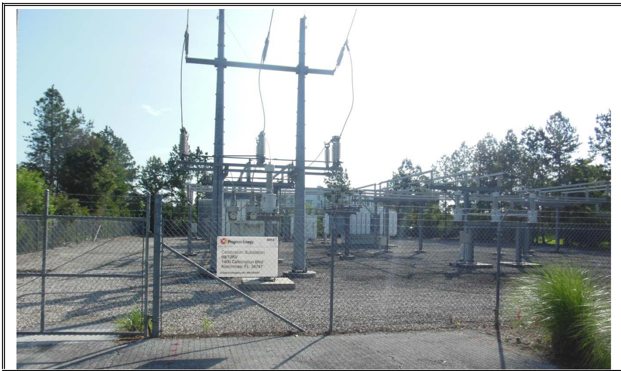
Site 19: Progress Energy Celebration Substation
