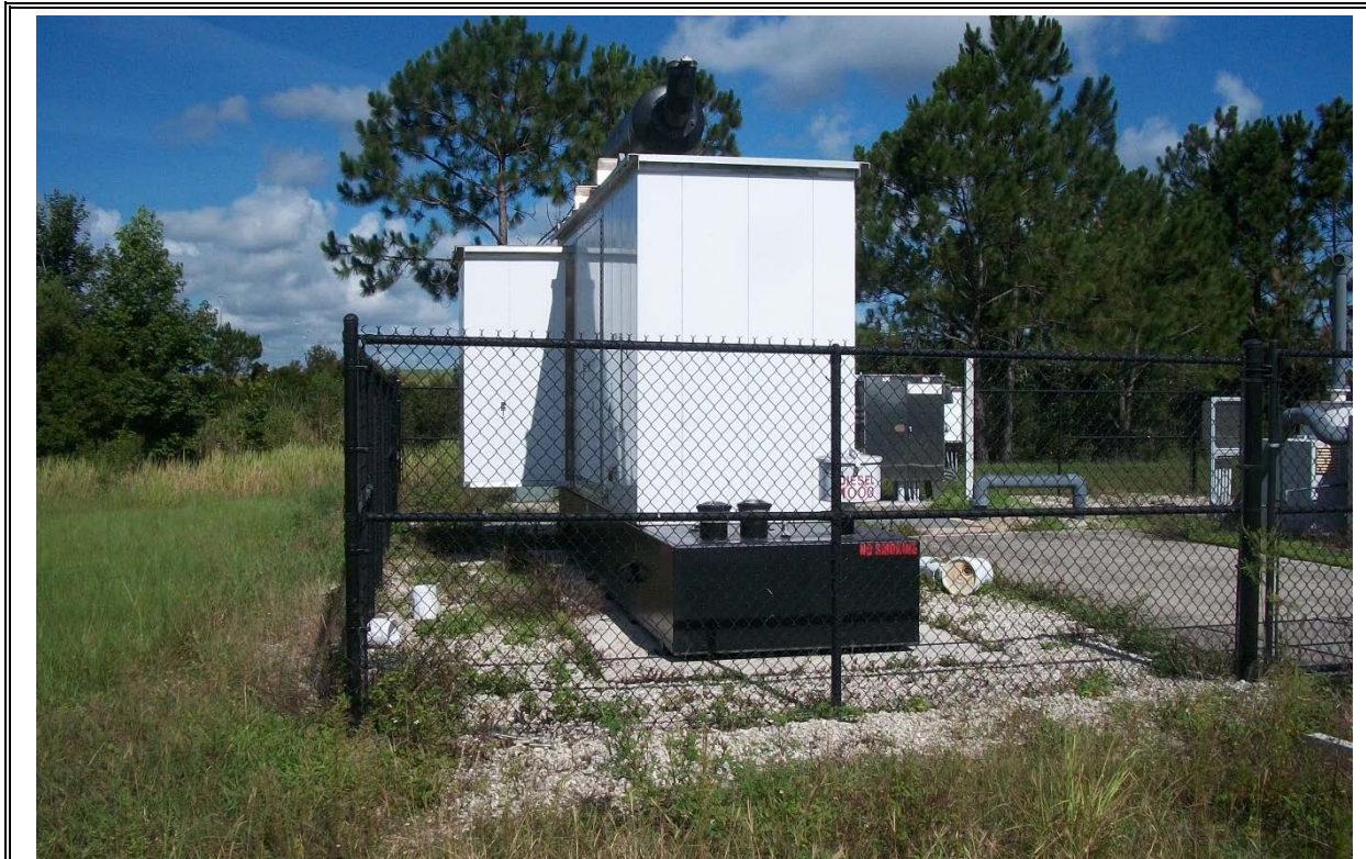
Site 18: Celebration Boulevard Lift Station #1
