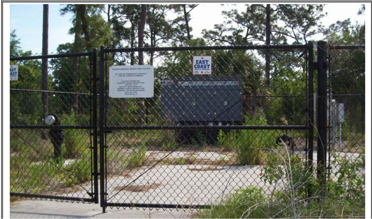
Site 37: Lift Station with Diesel Powered Emergency Generator
