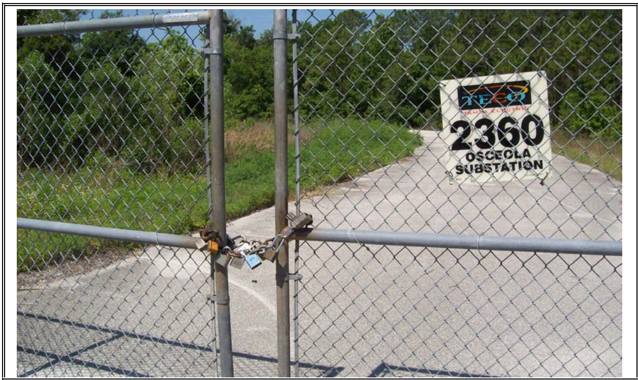
Site 17: TECO Substation #2360
