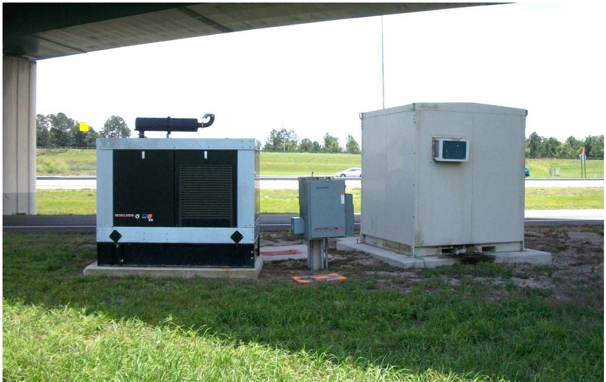
Site 24: FDOT Diesel Powered Emergency Generator B
