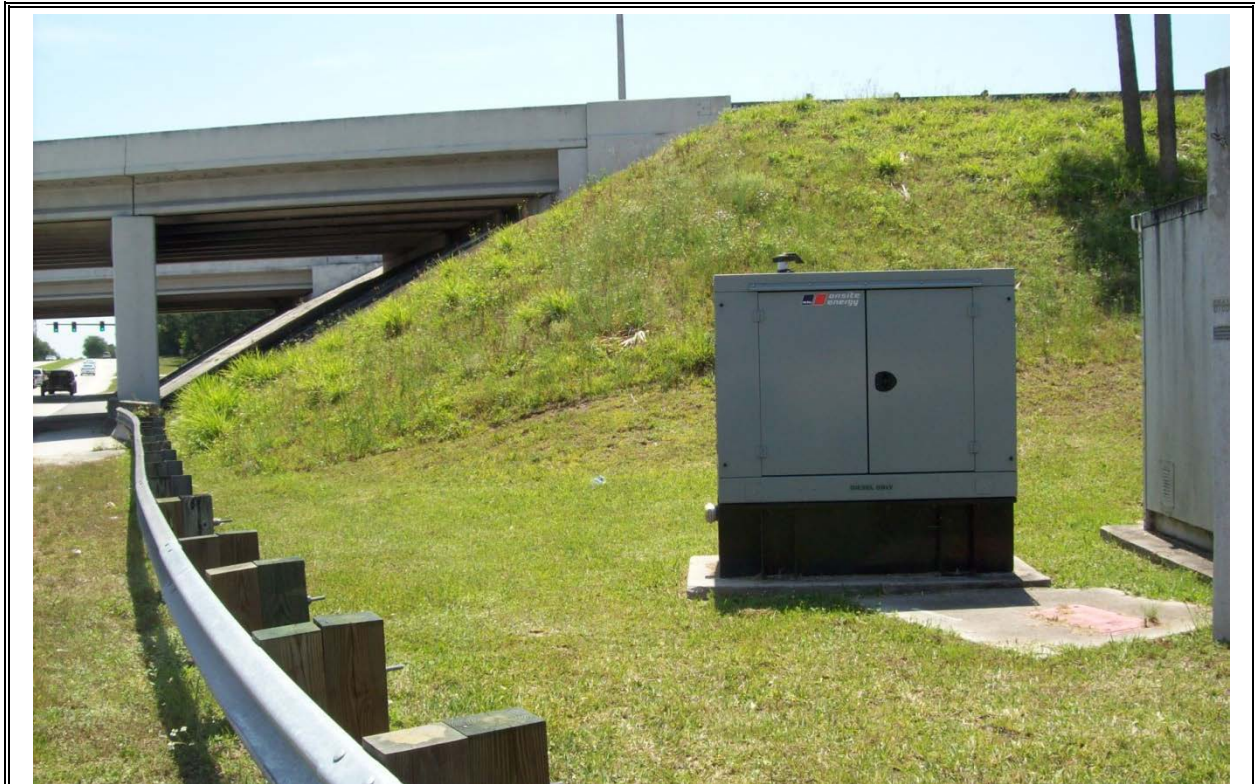
Site 3: FDOT Diesel Powered Emergency Generator A
