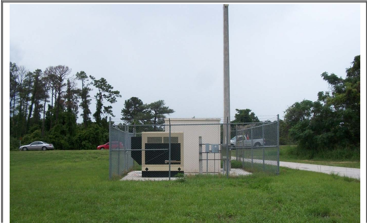
Site 85: FDOT Diesel Powered Emergency Generator B
