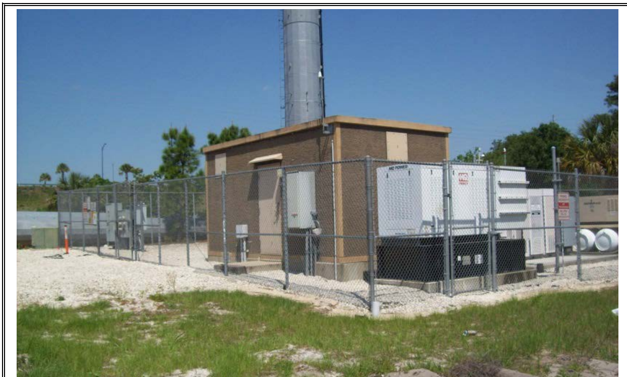
Site 11: Cell Tower with Diesel Powered Emergency Generator A
