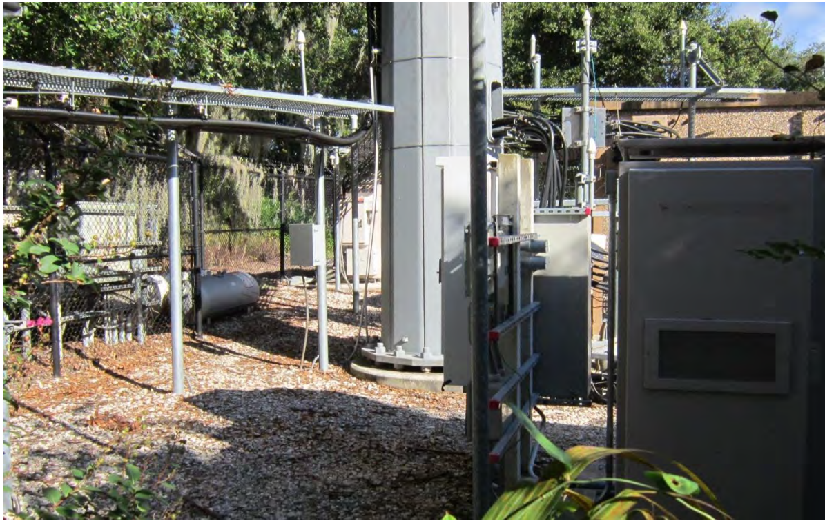
Site 158: Cell Tower with Natural Gas Generator C
