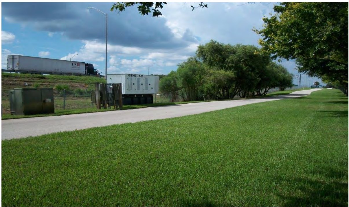
Site 154: Emergency Generator on International Parkway
