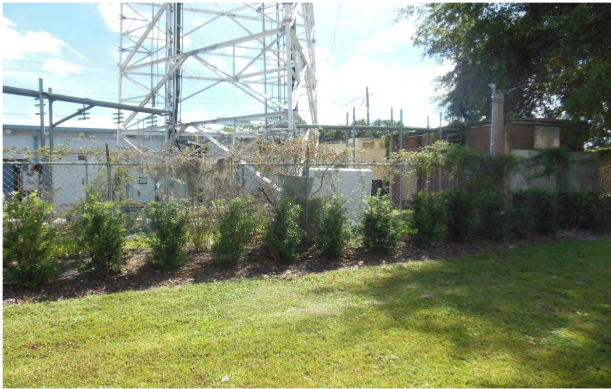
Site 254: Cell Tower with Diesel Powered Generator F
