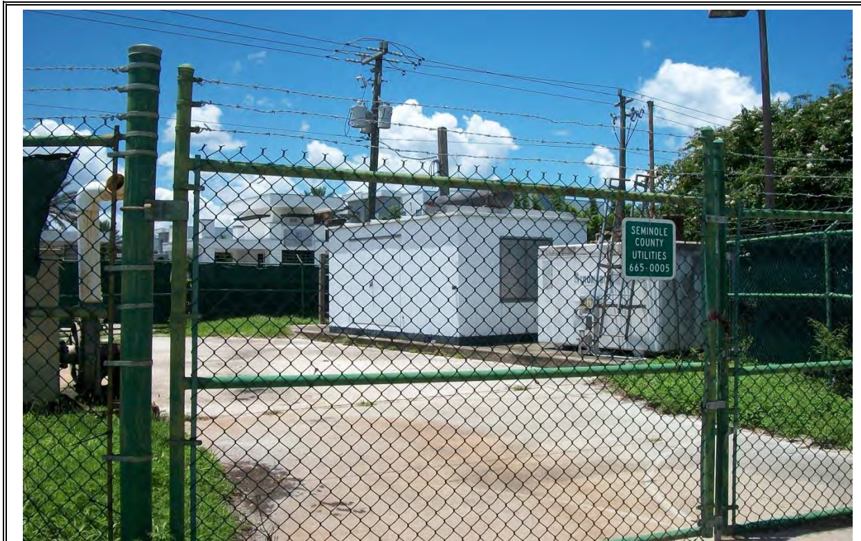
Site 168: Seminole County Utilities Generator
