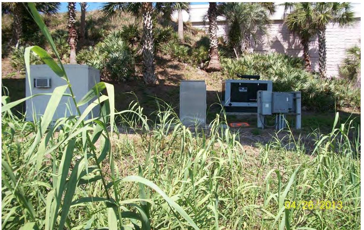
Site 290: FDOT Diesel Powered Generator
