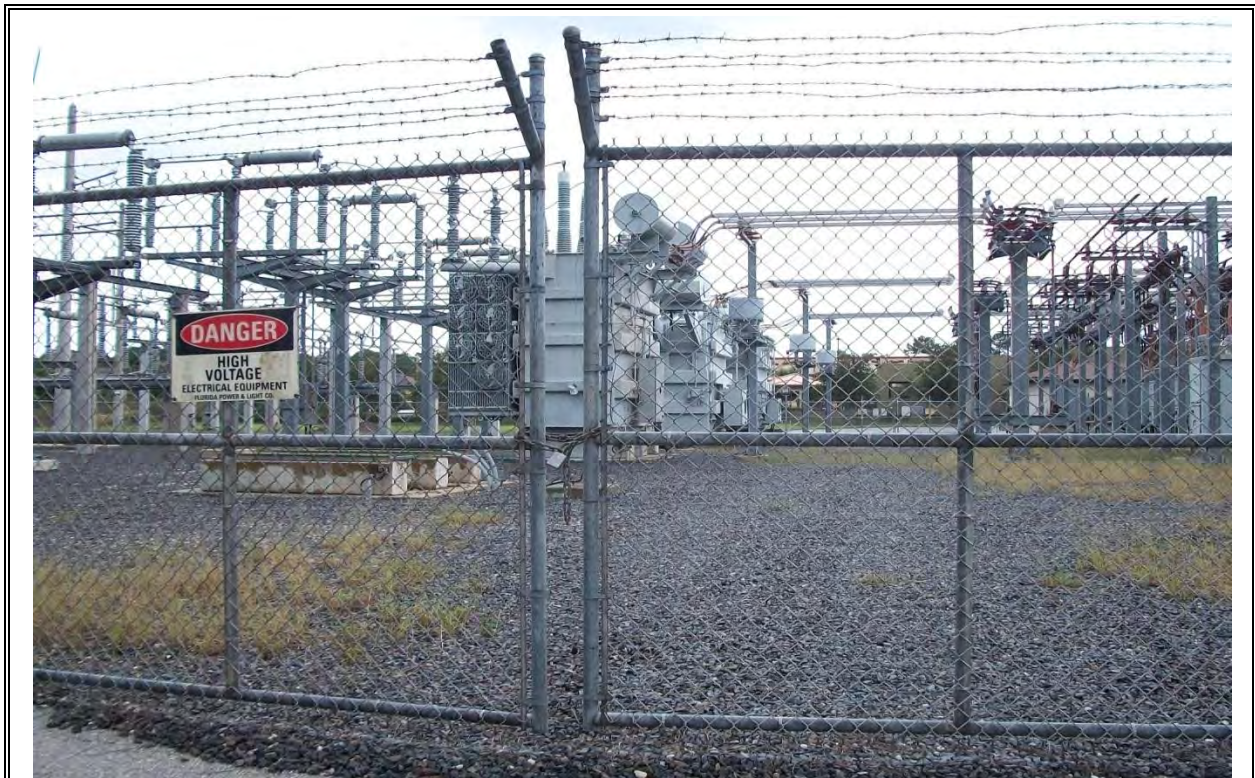
Site 215: FPL Rinehart Substation
