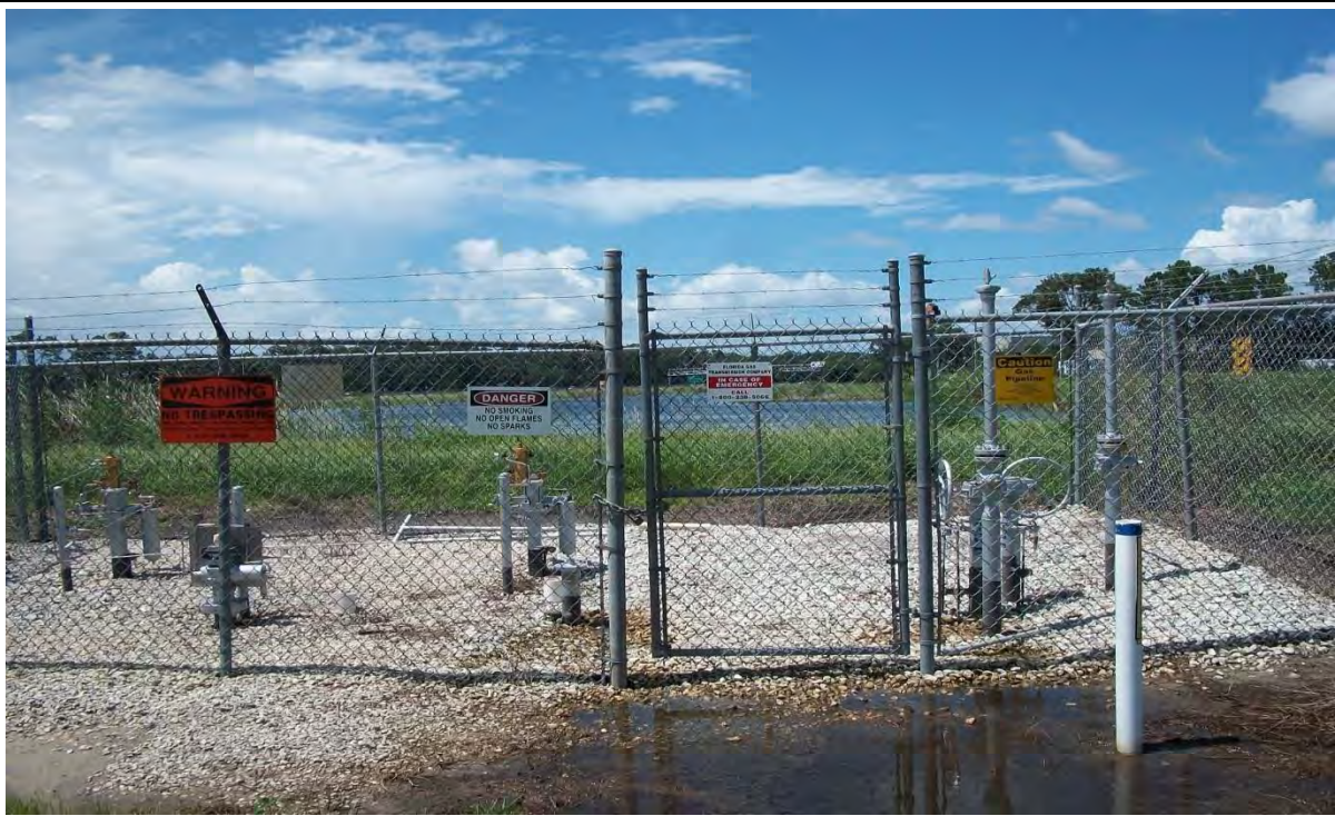
Site 241: Gas Facility at Andre Court
