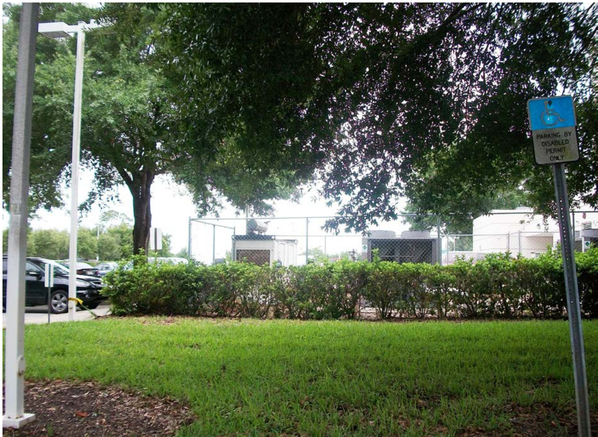
Site 36: Central FL Investments Inc. Sand Lake - generator
