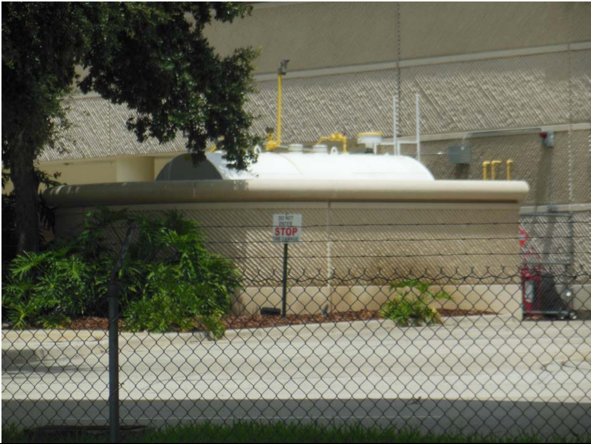
Site 18: Orange County Convention Center West Building – storage tank
