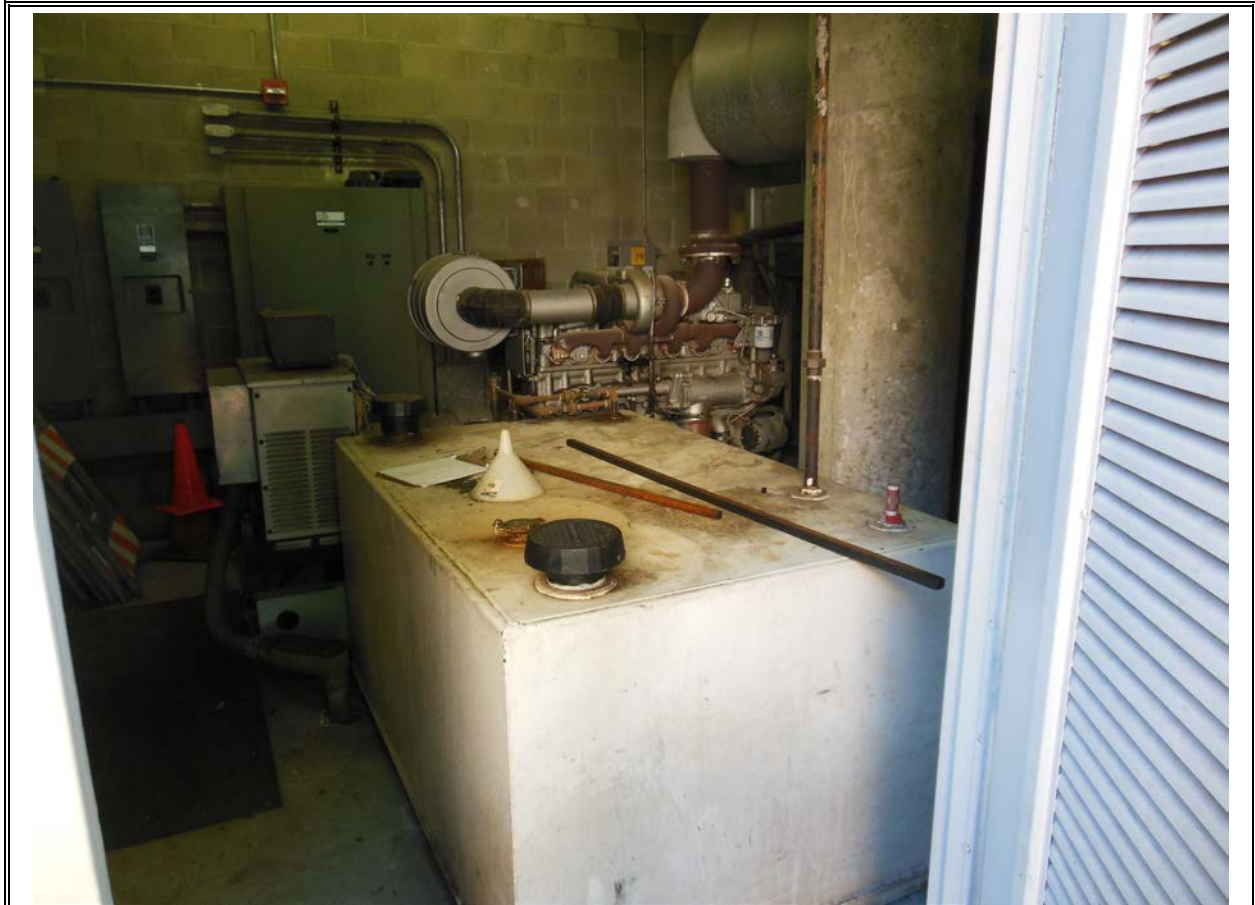
Site 55: Embassy Suites Hotel – diesel fueled generator
