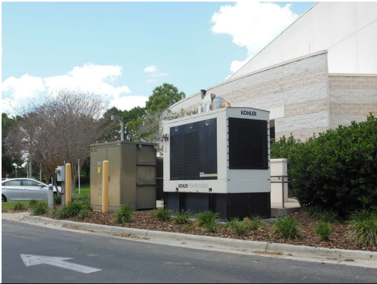
Site 92: Loews Hotels at Universal Studios Escape – diesel fueled generator
