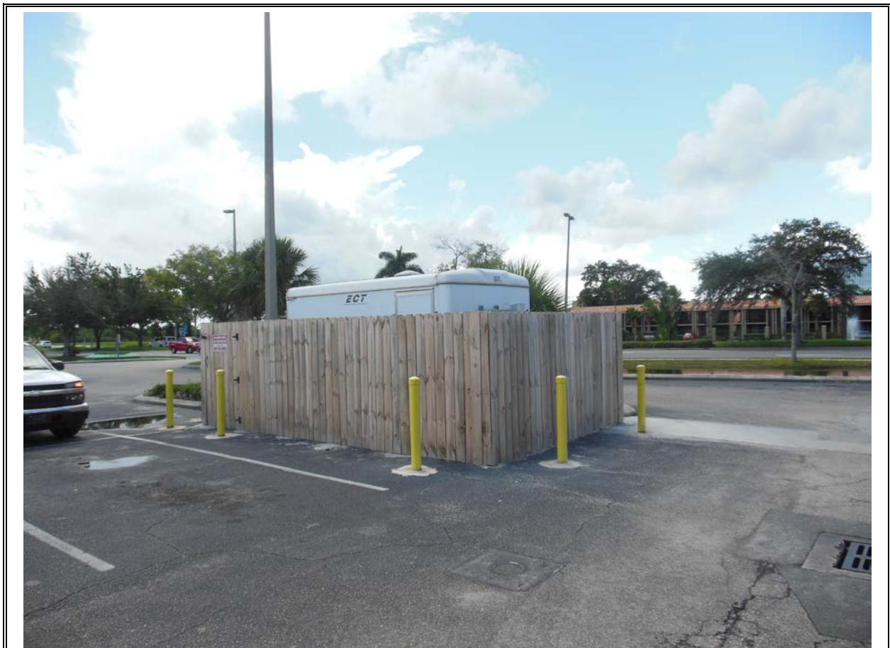
Site 13: Texaco Redmart – remediation system
