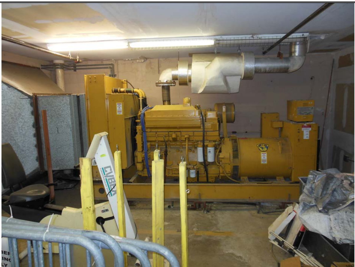
Site 50: Radisson Hotel – natural gas fueled generator
