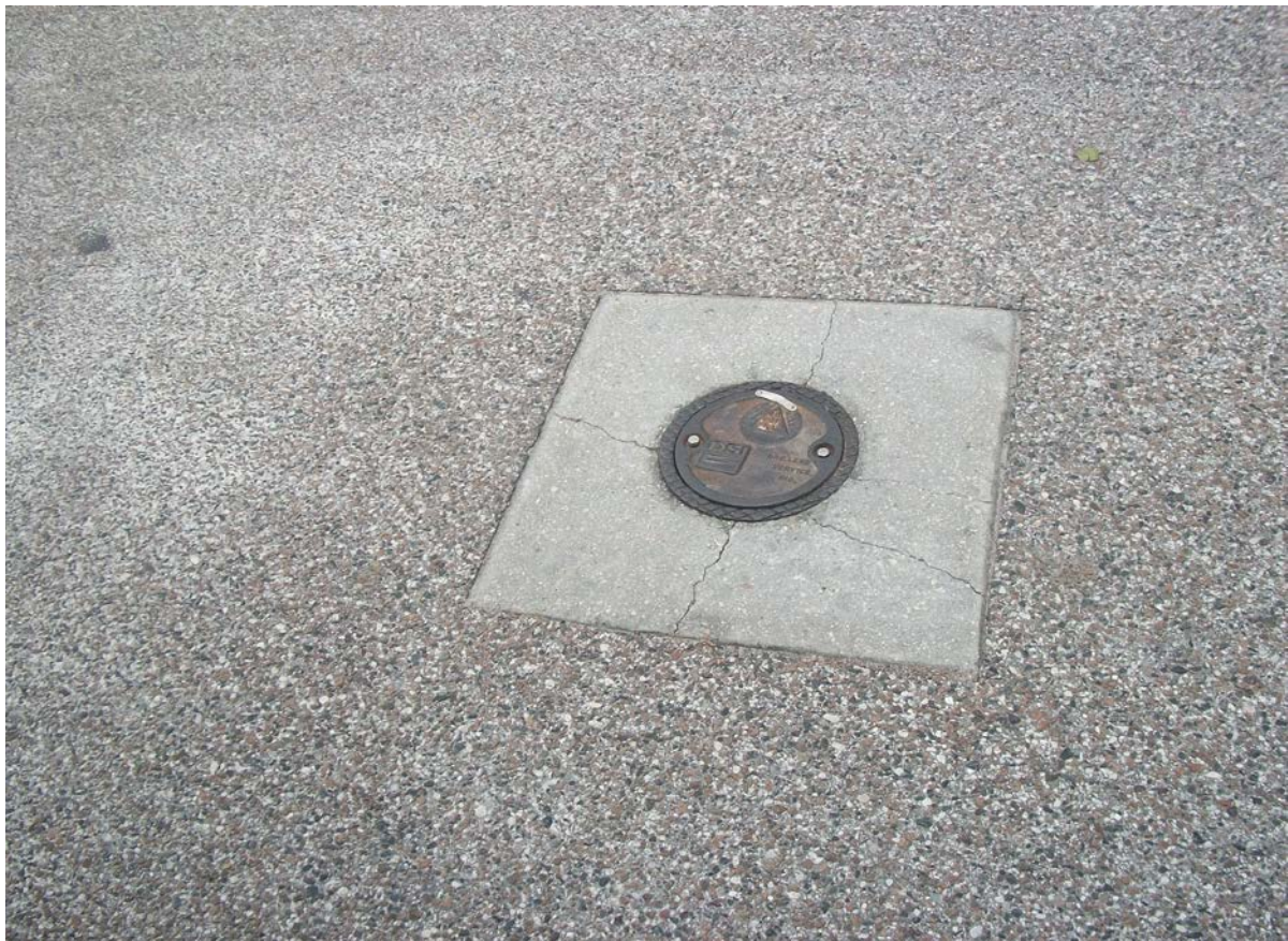
Site 65: Circle K #2708960 – monitoring well
