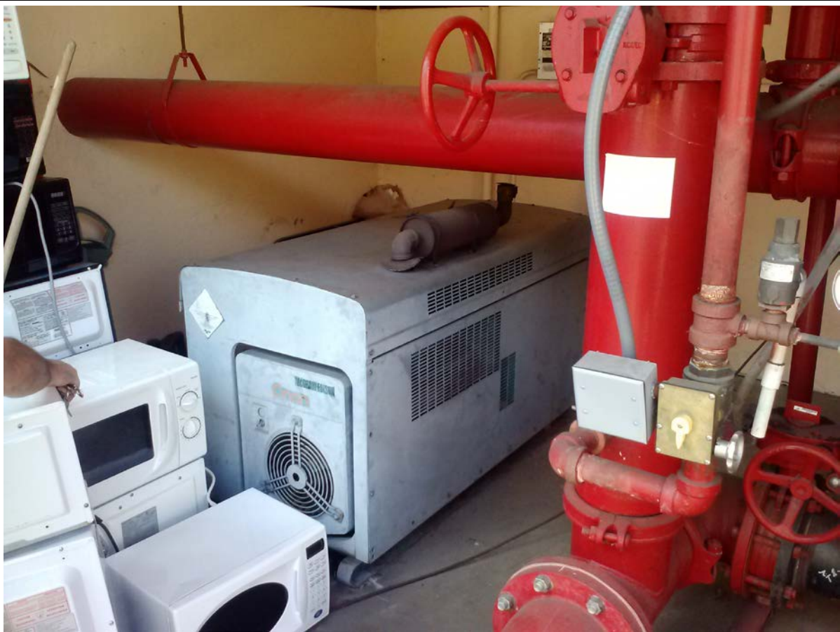
Site 41: Rosen Inn at Pointe Orlando - generator
