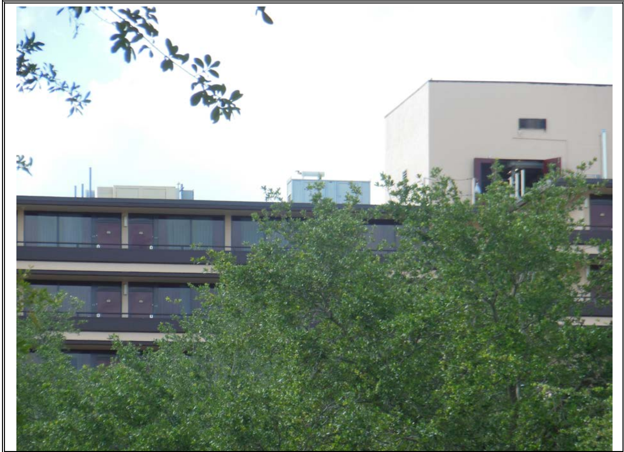
Site 41: Rosen Inn at Pointe Orlando - generator
