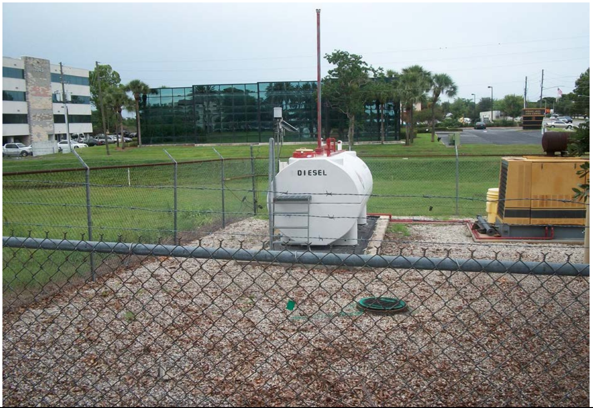
Site 68: Orange County Utilities Dr. Phillips PS #3151
