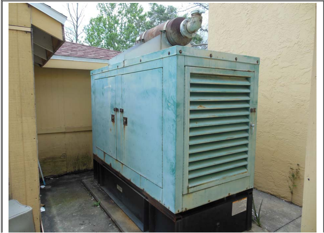
Site 45: Embassy Suites - generator
