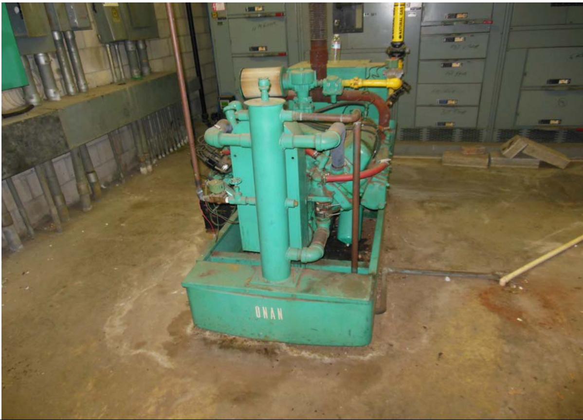
Site 97: International Palms Resort – natural gas fueled generator, northeast side of tower, inside maintenance room
