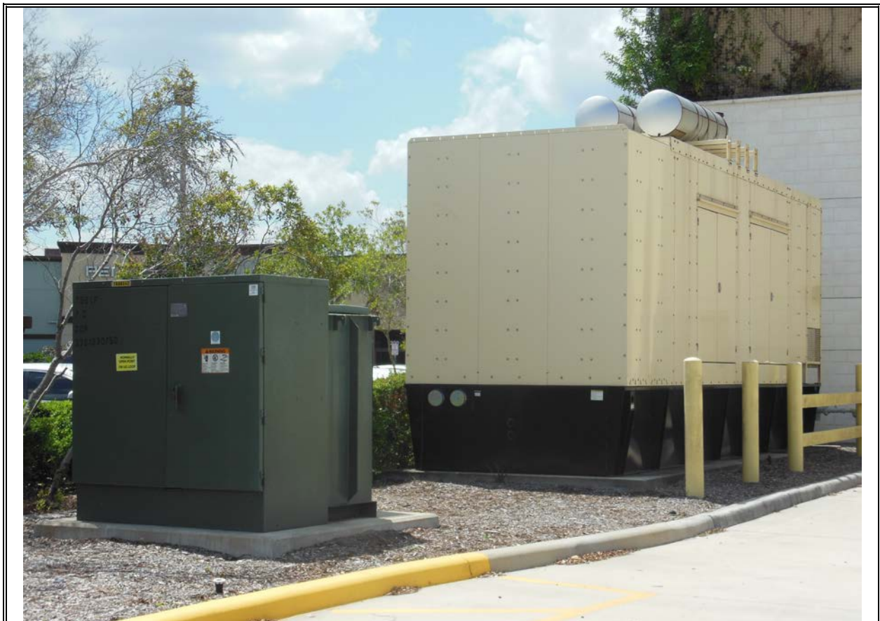
Site 61: Whole Foods Market Bay Hill – diesel fueled generator
