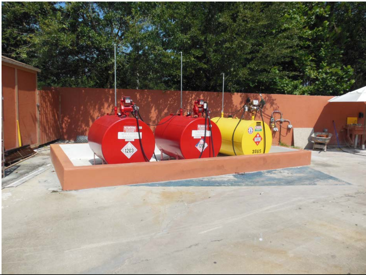
Site 23: Westgate Lakes Resort and Spa – storage tanks
