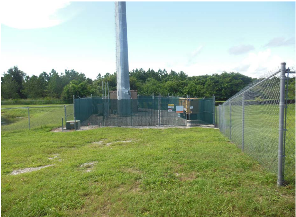
Site 60: Cell Tower with Diesel Fueled Generator B
