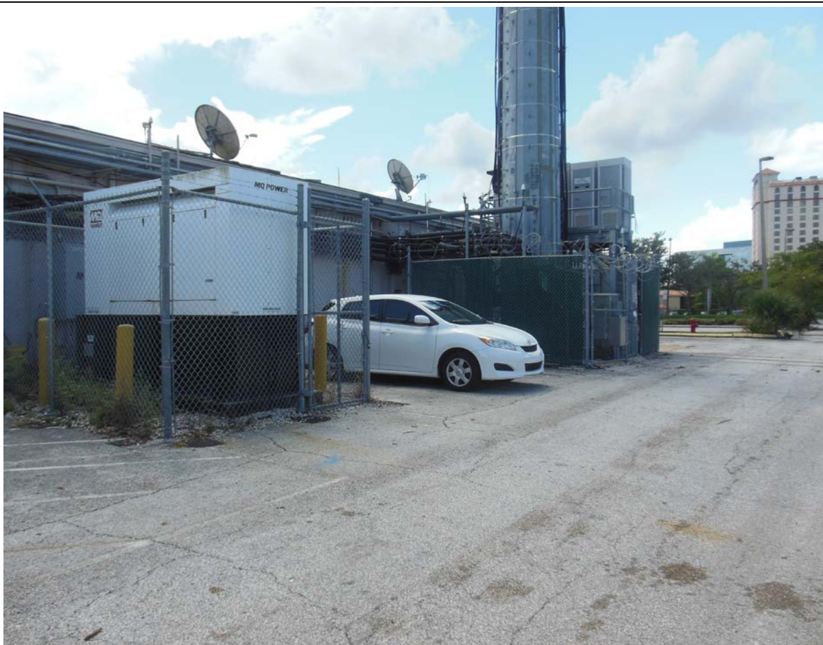
Site 12: Cell Tower with Diesel Generator A
