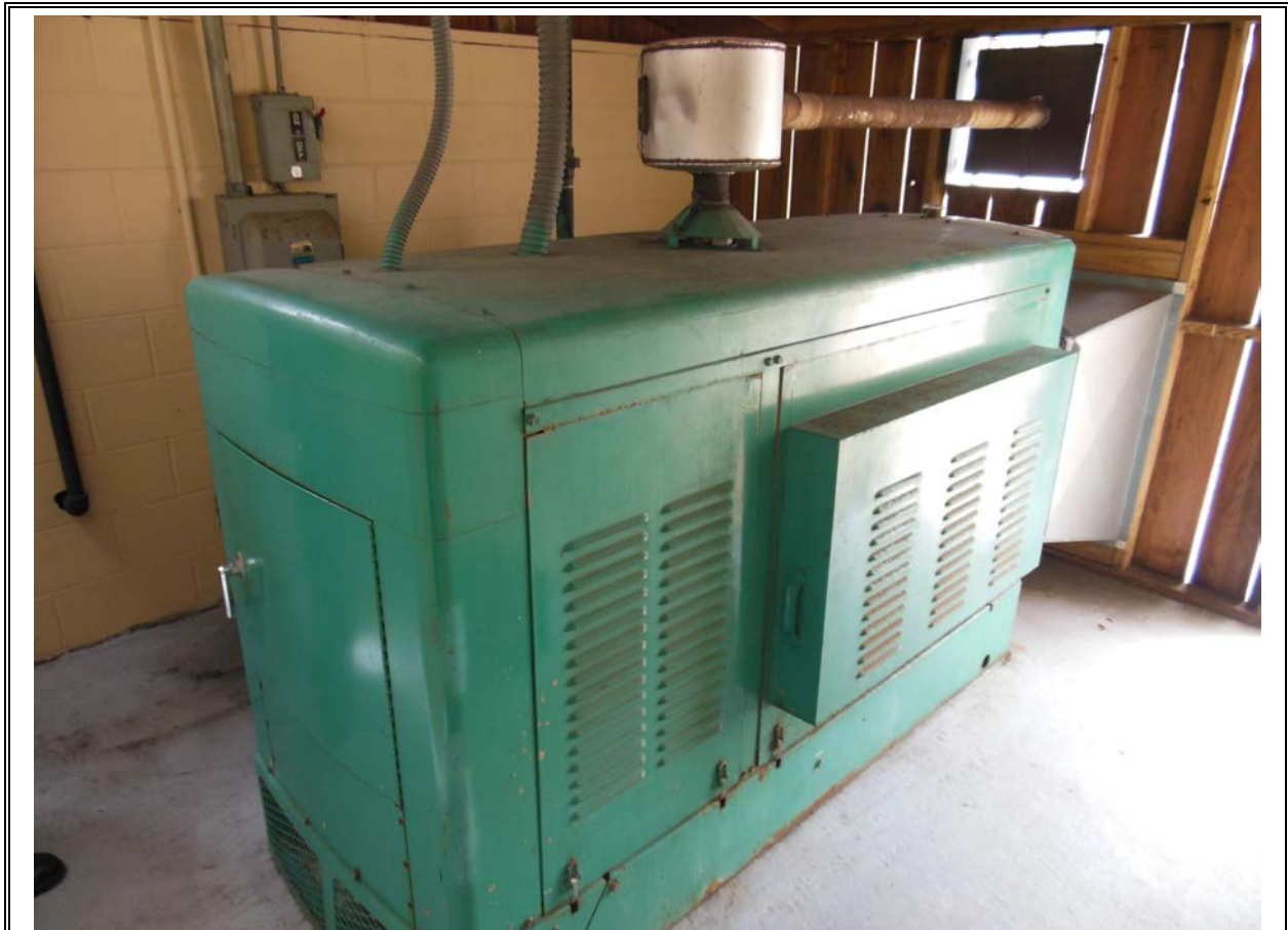
Site 80: Quality Inn International – natural gas fueled generator
