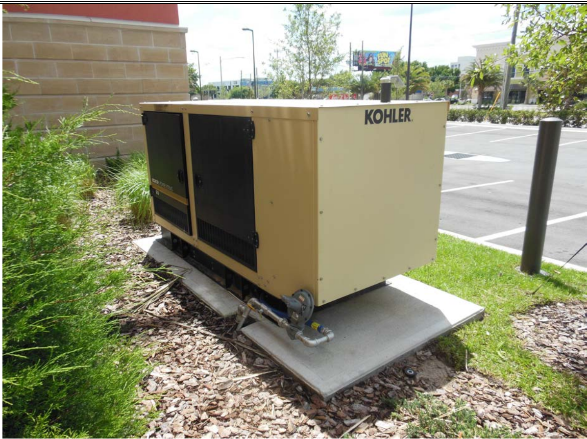
Site 77: Drury Inn Hotel – natural gas fueled generator
