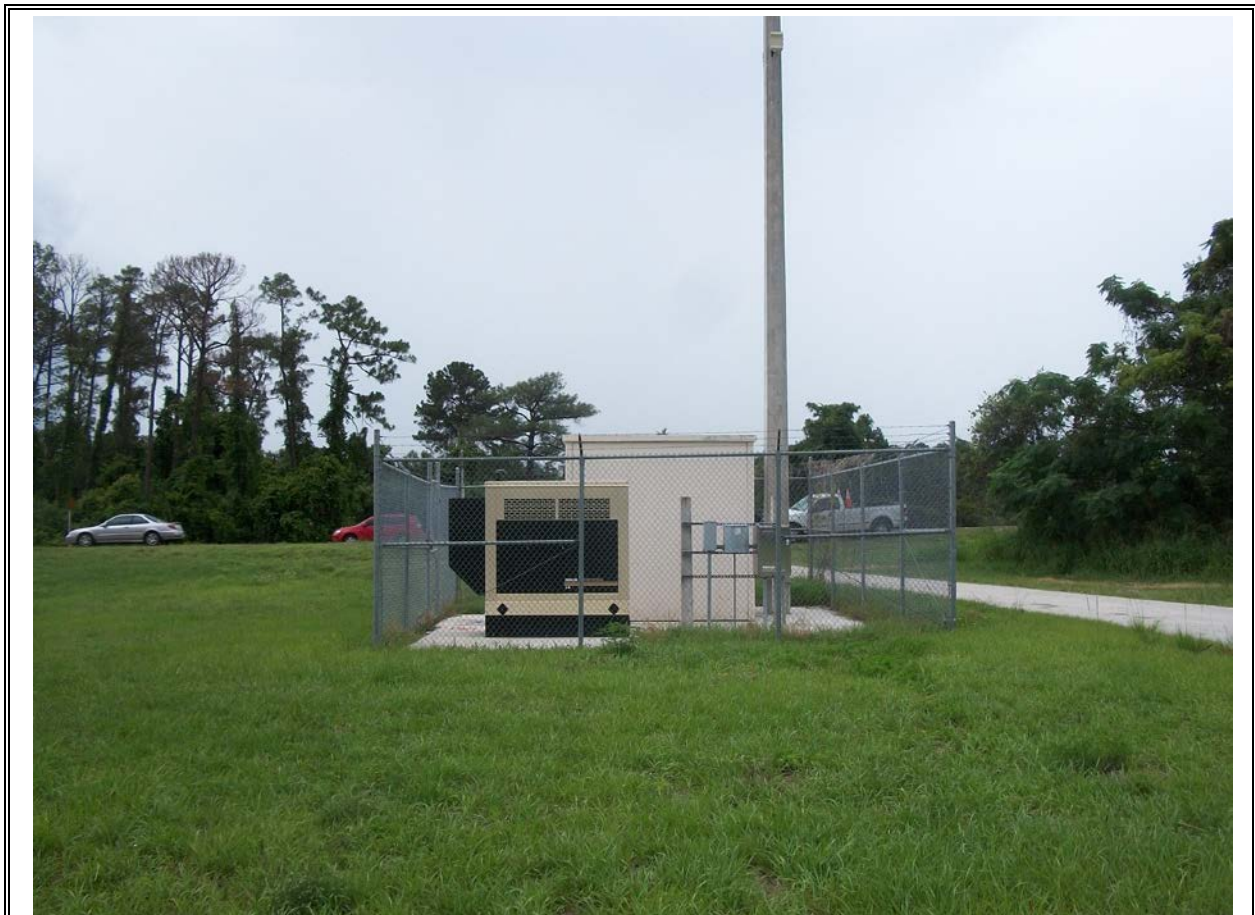
Site 16: FDOT Diesel Power Generator A
