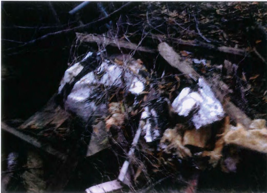
18. View of homogeneous area BDP1-3, heating, ventilation, and air conditioning (HVAC) duct mastic located in Building Debris Pile #1. Laboratory analytical results showed 8% chrysotile asbestos in homogeneous area BDP1-3.
