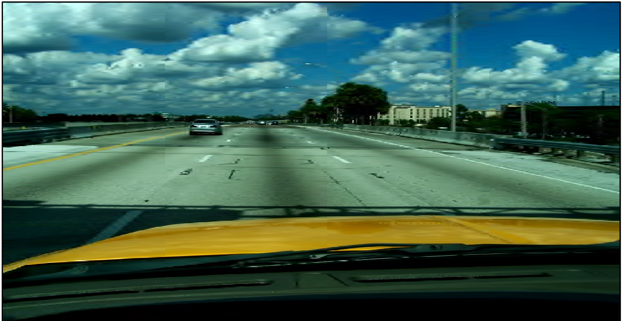
Photo 8: I-4 eastbound near MP 8.250. The approaches to the bridges within the project limits are in fair condition. Corrective actions will not be needed.
