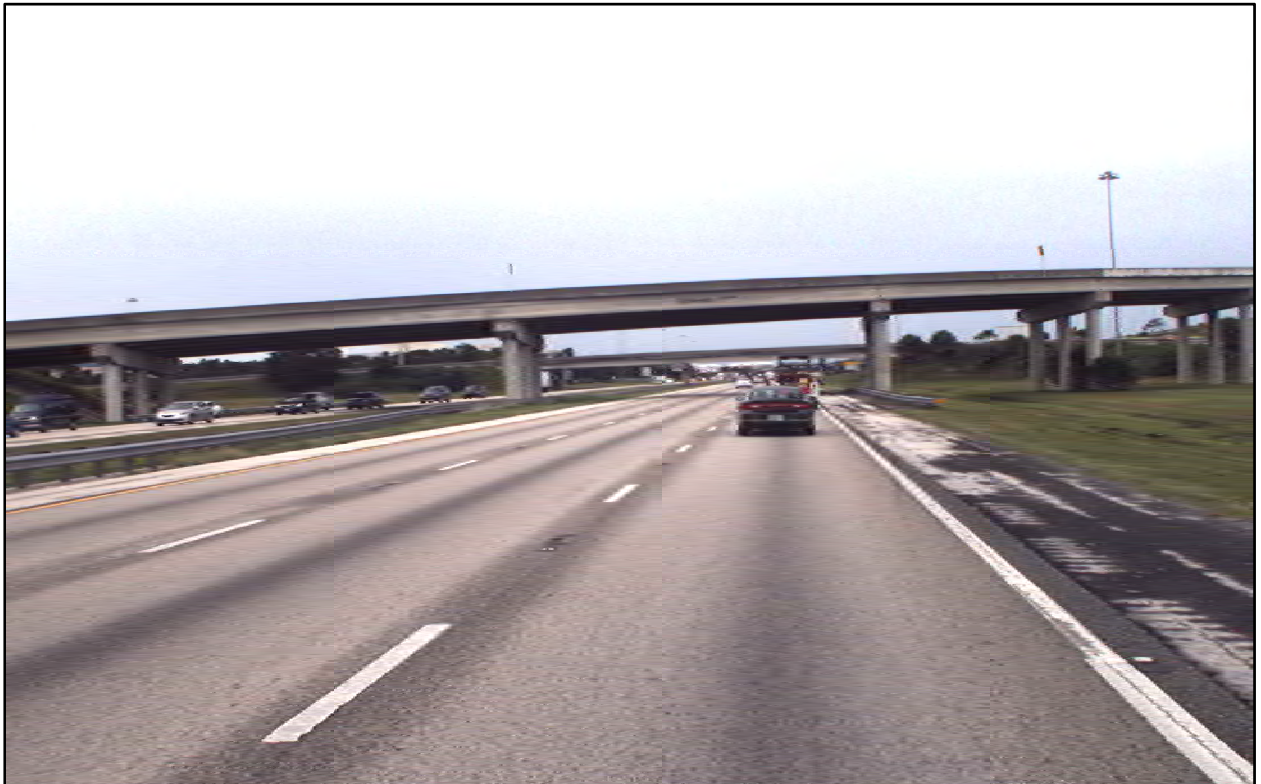
Photo 2: I-4 westbound near MP 6.430. The westbound outside shoulder from MP 6.200 to MP 6.430 was repaired with what appear to be chip seal that has raveled with time.
