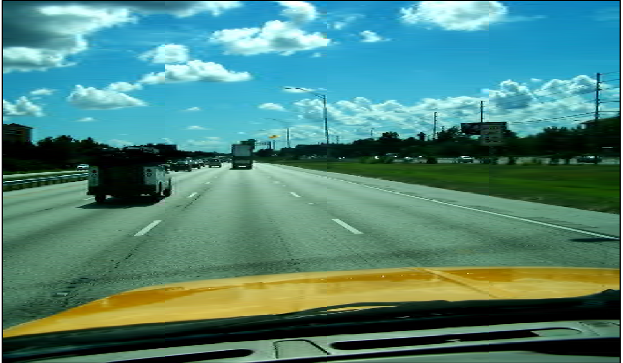
Photo 5: I-4 westbound near MP 7.593. This photo shows that the westbound mainline lanes have less severe pavement distress than the eastbound lanes.
