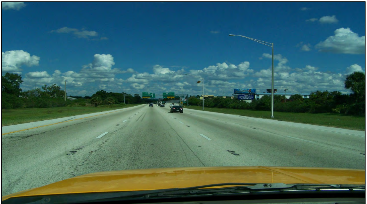
Photo 10: I-4 eastbound near MP 9.155. The eastbound roadway from MP 8.844 to the end of the project at MP 9.249 was last resurfaced in 1993 and is in very worn condition.
