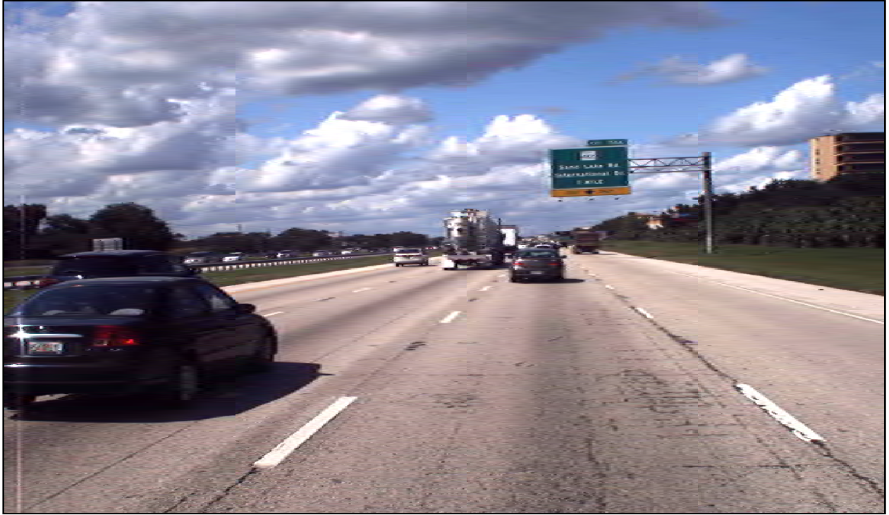
Photo 3: I-4 eastbound near MP 6.885. This is an example of the poor condition of the R3 lane with the cracking in the outside wheelpath.
