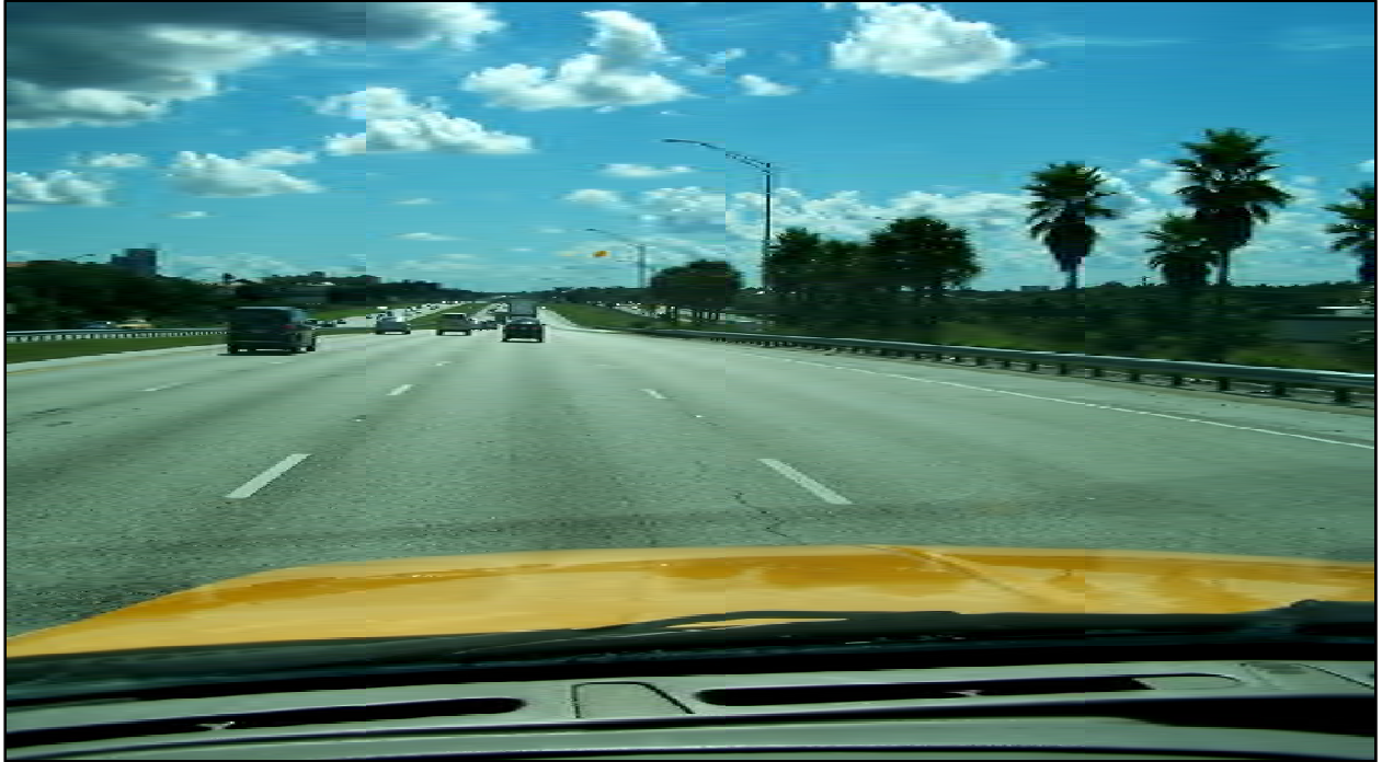
Photo 7: I-4 westbound near MP 8.198. The westbound mainline lanes have less cracking distress than the eastbound roadway.
