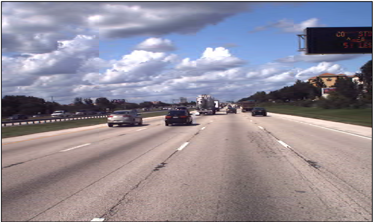
Photo 4: I-4 eastbound near MP 7.235. This is another example of the severe cracking in the outside wheelpath. This is also an area where the Ground Penetrating Radar indicates thinner pavement averaging 6.6 inches.
