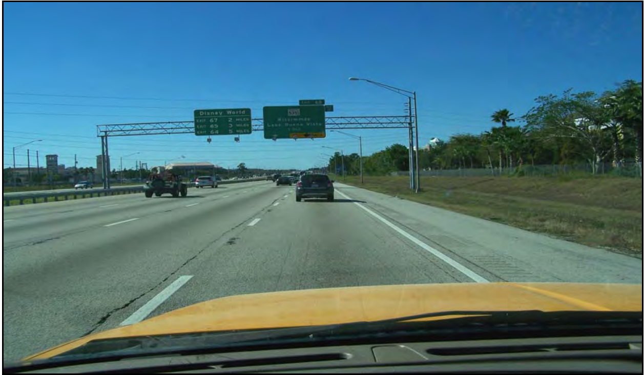
Photo 7: I-4 westbound near MP 3.930. There is a longitudinal crack between the L3 and L4 along a construction joint.
