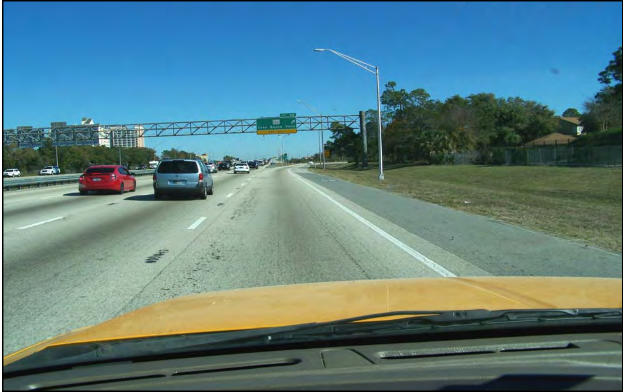
Photo 1: I-4 eastbound near MP 2.089. From the beginning of the project at MP 1.740 to where the R4 lane ends at MP 2.130 there is a continuous series of alligator cracks and raveling in the inside wheelpath. This is also where a significant amount of traffic going to local attractions departs I-4.
