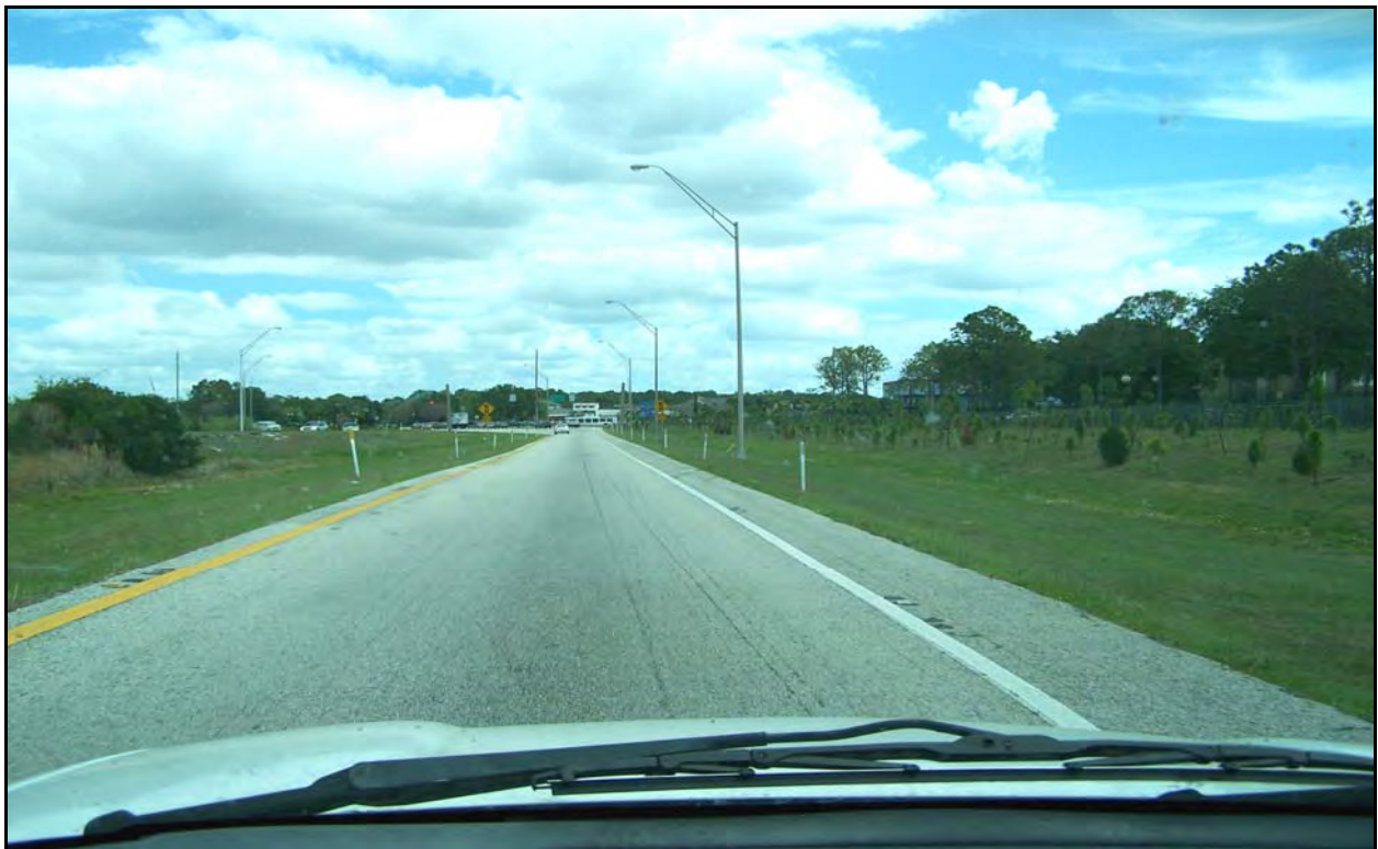
Photo 10: Ramp 080 from I-4 Eastbound to SR 535. The ramps for the SR 535 are in fair condition with few distresses.
