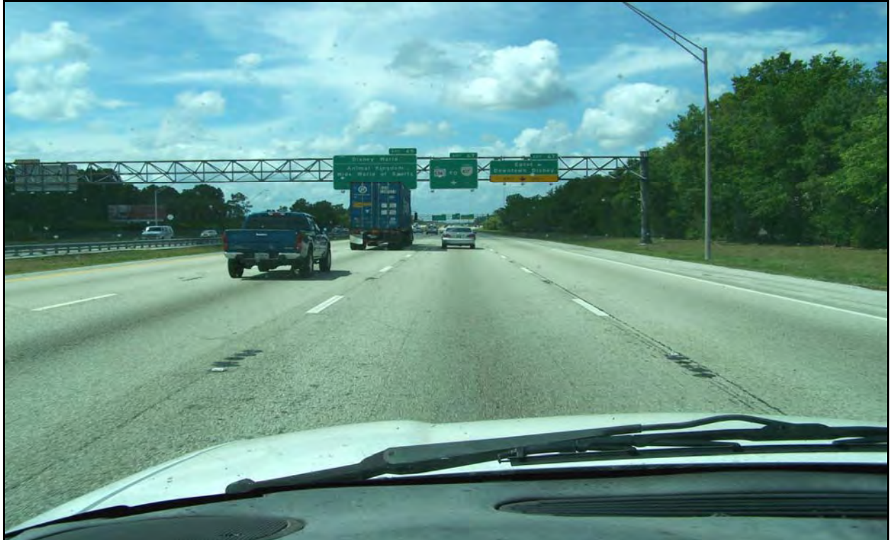
Photo 6: I-4 westbound near MP 2.193. The westbound roadway has light pavement distresses. Note the pop-up of aggregates in the open-graded friction course in the L3 lane.
