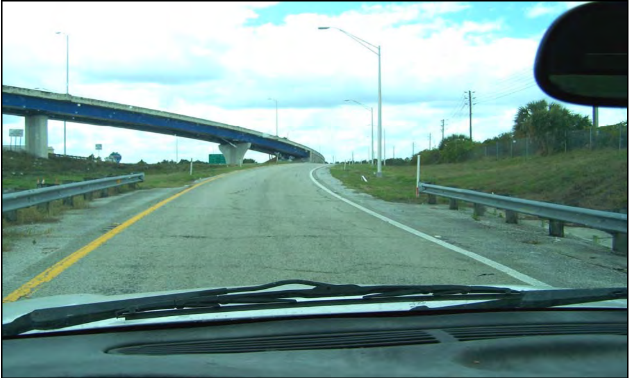
Photo 11: Ramp 021 from Central Florida Parkway to I-4 Westbound. The ramps at the interchange with the Central Florida Parkway are in poor condition. Note the severe cracking and raveling distresses.
