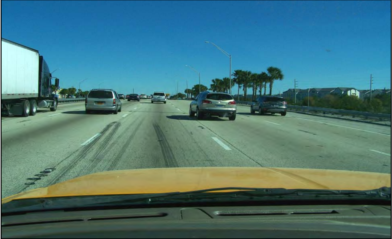
Photo 3: I-4 eastbound near MP 2.484. The inside R1 and R2 lanes of the eastbound roadway have far fewer pavement distresses than the R3 and R4 lanes.
