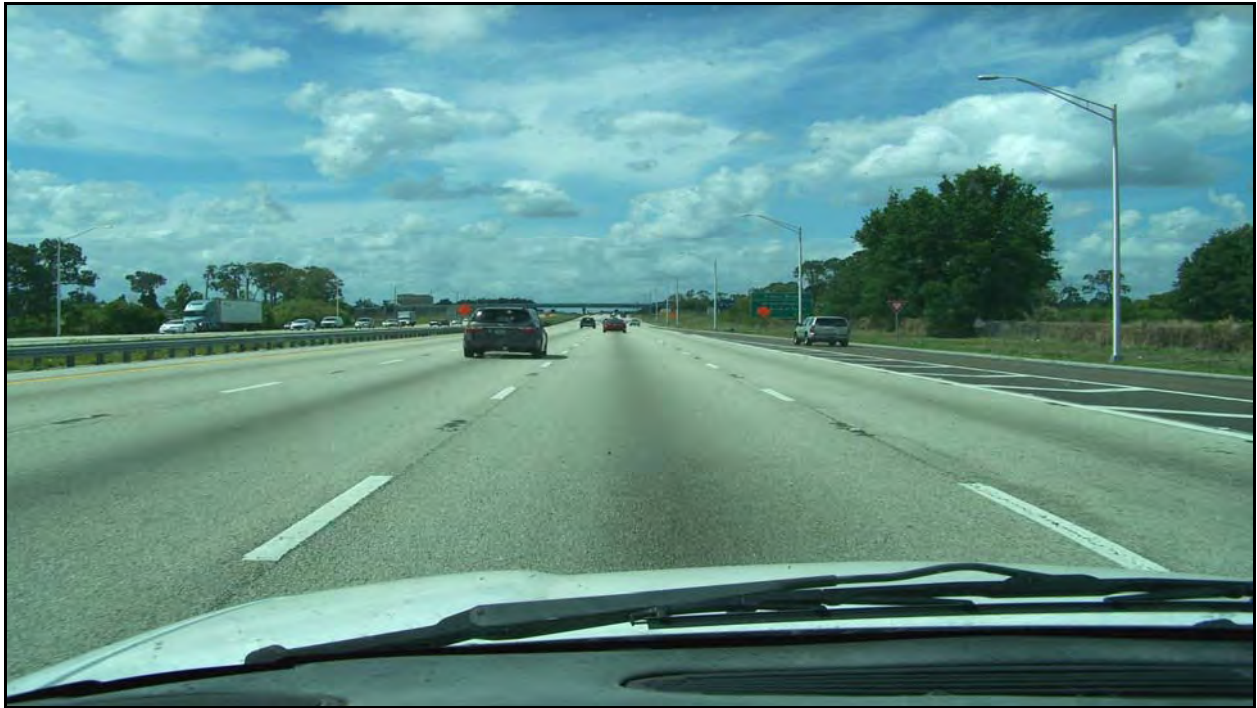
Photo 8: I-4 westbound near MP 4.903. Typical condition of the westbound roadway.
