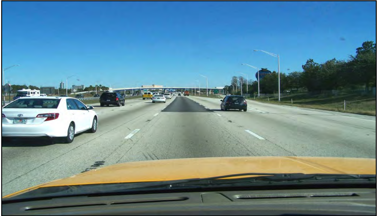
Photo 5: I-4 eastbound near MP 5.124. There are a number of patches that have been placed in both roadways to repair ride or raveling problems.
