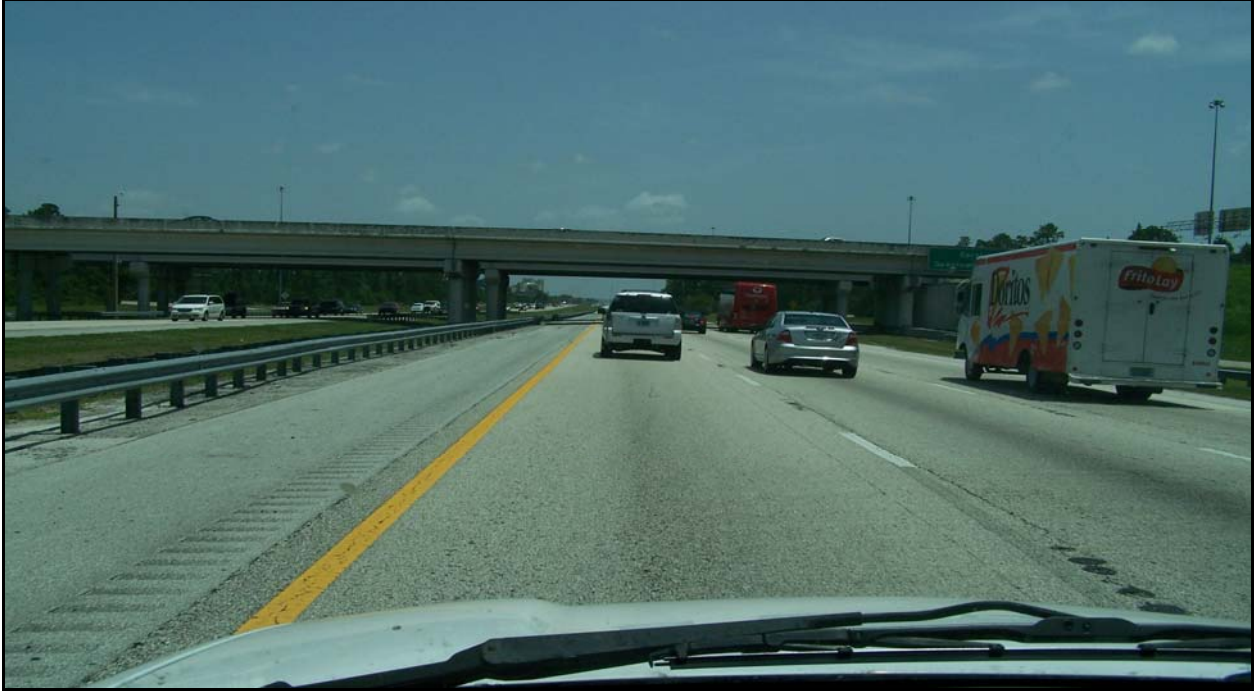
Photo 3: I-4 eastbound near MP 1.049. This photo shows the fair condition of the inside paved shoulder and the R1 lane.
