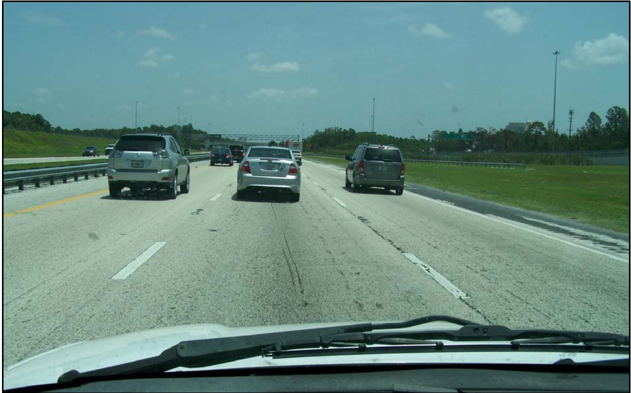
Photo 2: I-4 eastbound near MP 0.454. The R1 and R2 lanes are in better condition than the R3 travel and R4 auxiliary lanes. Note the chip seal overlay on the outside shoulder.
