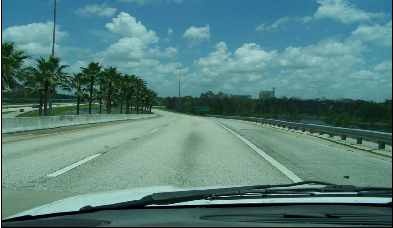
Photo 7: I-4 eastbound on Ramp 75039-008. This is the ramp from I-4 eastbound to SR 536 westbound. Note the lack of pavement distress other than oxidized friction course.
