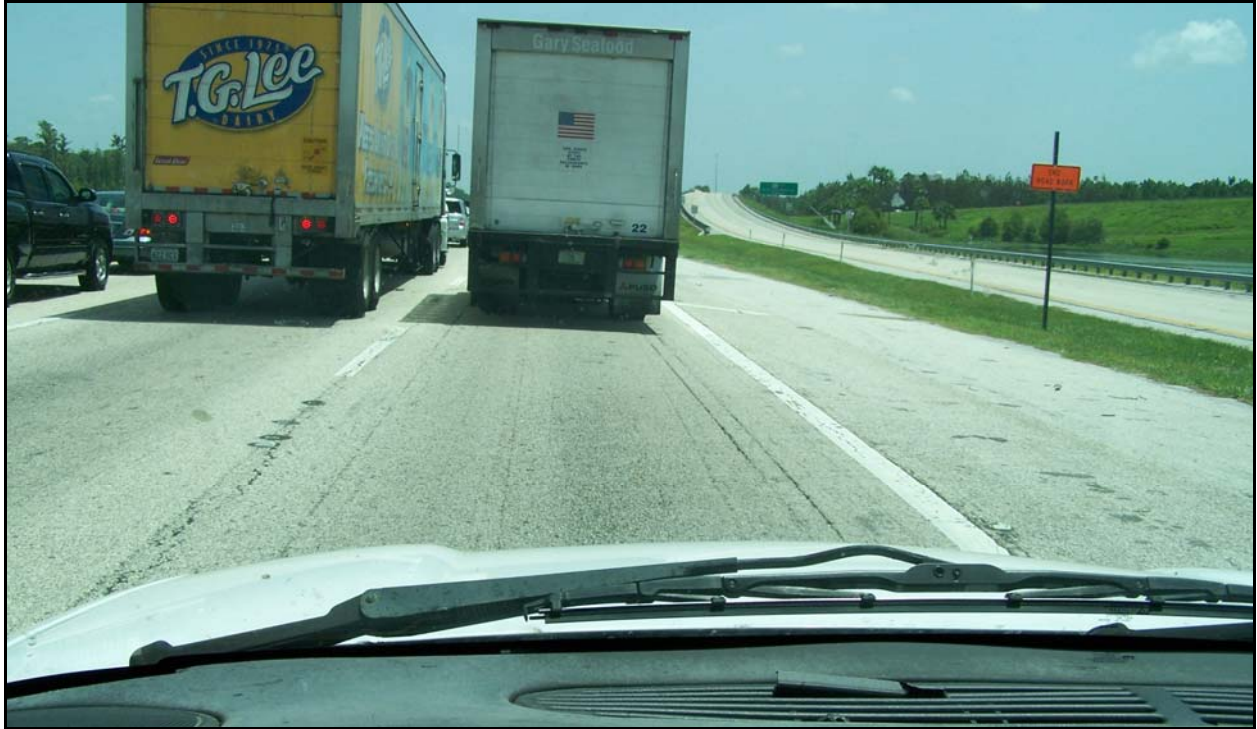
Photo 1: I-4 eastbound near MP 0.029. This photo shows the deteriorated condition of the R3 lane.
